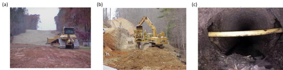
Figure 2.4. (a) Bulldozer grading prior to pipeline burial. (b) Pipeline trenching operations. (c) Example of a problematic cross bore of a gas pipeline through a sewer line.
